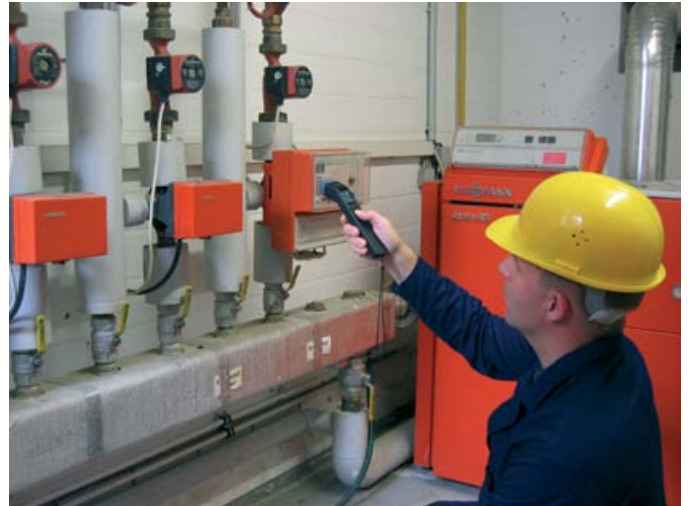
Checking the temperature of heating circles
